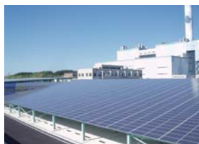
2006 Dong-hae PV Power Plant
