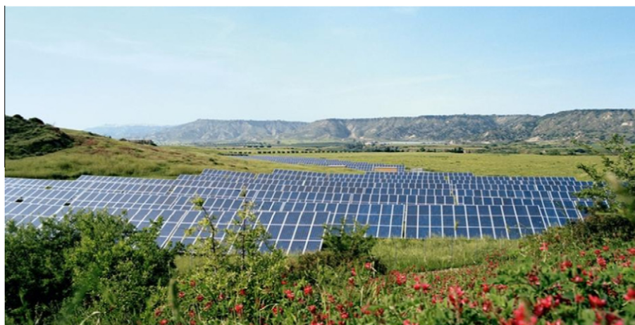
Fig. 3. One of the two monitored PV plants.
